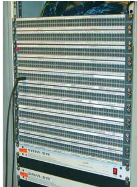
Multimedia control room, Hotel Estrel, Berlin, Germany
