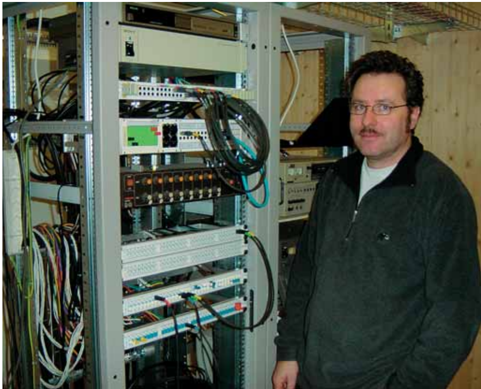
Main switch room at AVMedia Ltd., Zollbrück (Switzerland), owner Mr. Beat Lüthi
