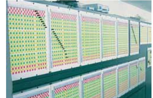
Loudspeaker distribution at Jahrhunderthalle Bochum, Germany
