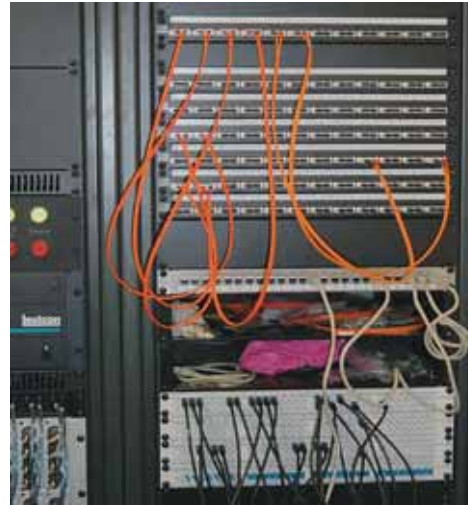
Digital, analogue and fibre optic patch panels
