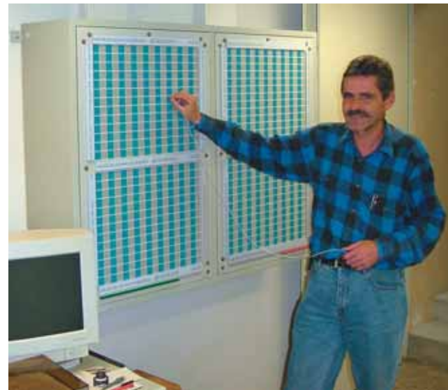
Telecom Matrix: GKV 208x288 341 SS K, Swiss Telecom
